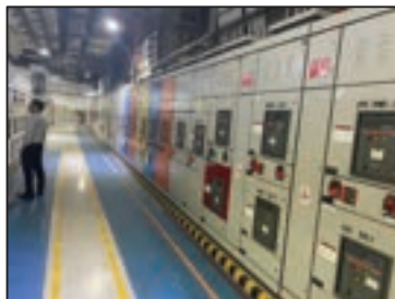
View of LT Panel Room
