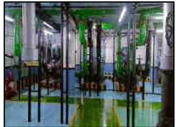
View of Generator Room
