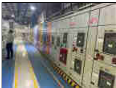
View of LT Panel Room
