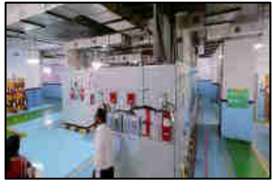
View of Electrical room
