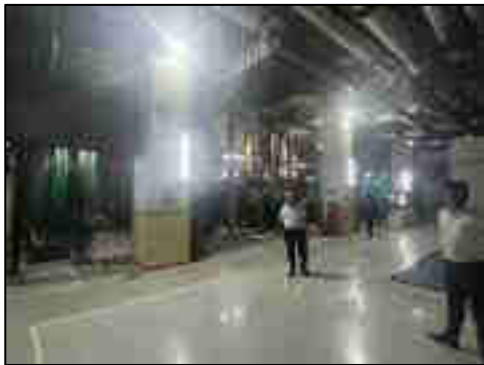
View of DG Room
