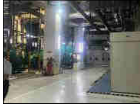
View of LT Room
