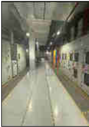
View of DG Room Tower 4 ,5 & 6
