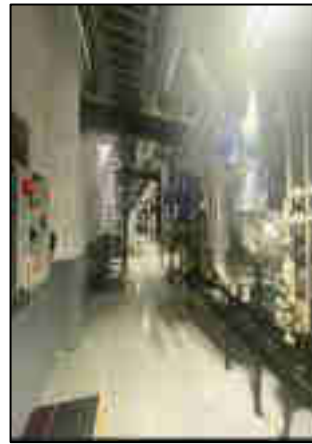
Internal View of Plant Room Tower 4, 5 & 6
