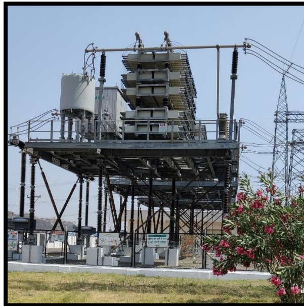
Fixed Series Capacitor
