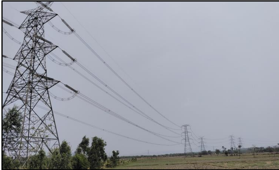
Angle Tower of 765 kV Transmission Line
