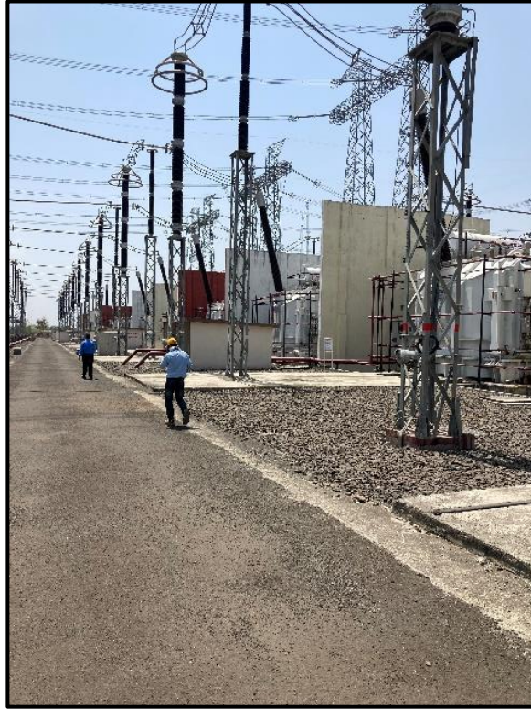
Inter Connected Transformer (ICT) – 7 x 500 MVA
