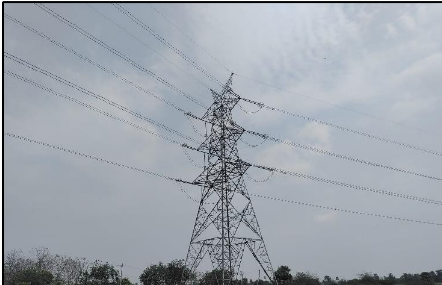
Angle Tower of 400 kV Transmission Line
